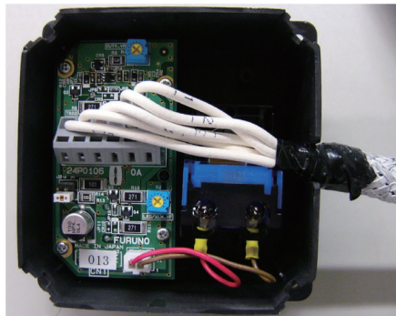
2) Process cable and connect cable to WAGO terminal block. Use terminal opener (inside Processor Unit) to open terminals. (Shown: Timer Reset Panel)
