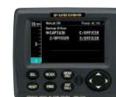
Main Alarm Panel
