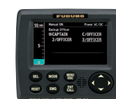
Main Alarm Panel
